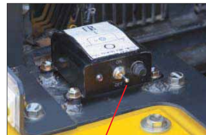
Electric priming pump switch
